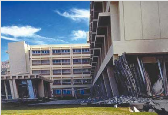
Damage to hospital in 1971 San Fernando Earthquake
